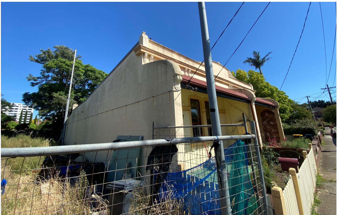
Figure 5 The roof line behind the parapet of 11 Archer Street. The architrave details of the windows is also visible. (Source: HAA)
