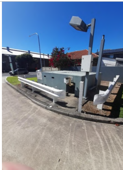
Photo 10: Bunded above ground LPG tank on the 7-Eleven Petrol Station forecourt.
