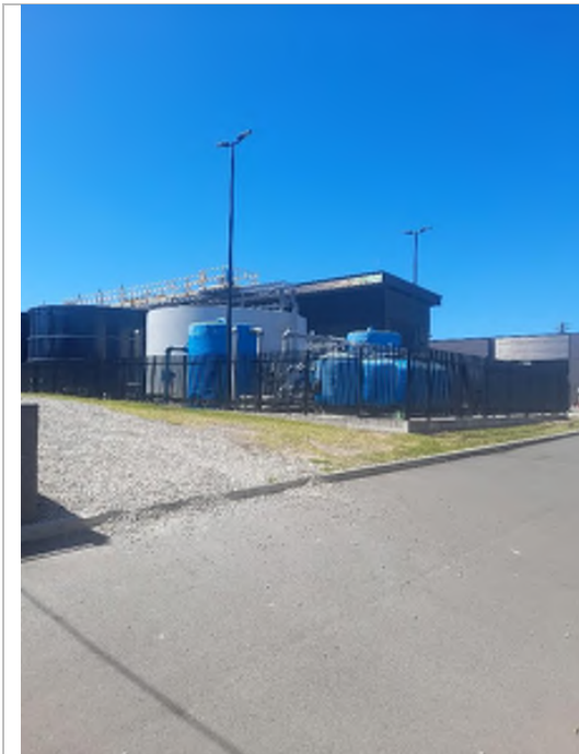
Photo 17: WestConnex M4 groundwater treatment plant. View looking south-east from Gipps Street.
