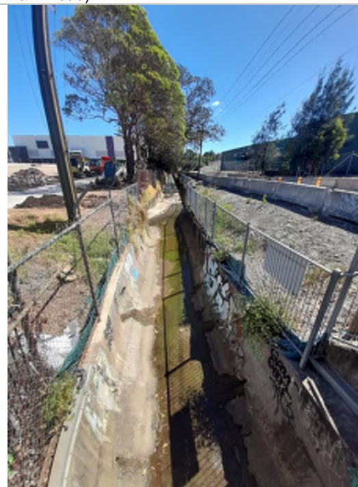
Photo 16: St Lukes Canal showing weepholes and cracks. Photo taken from Parramatta Road looking north.
