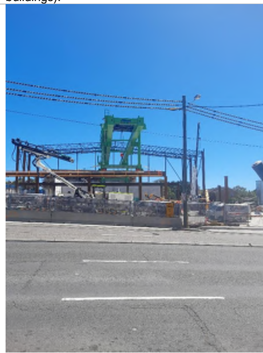
Photo 20: Construction of the Burwood North Metro Station on the corner of Parramatta and Burwood Roads).
