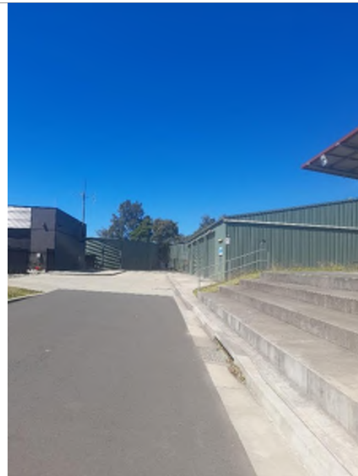
Photo 18: City of Canada Bay Council treatment and water storage tanks (green buildings).
