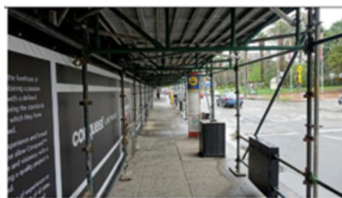
Example 16: Scaffolding Style – Not Acceptable in any zones
