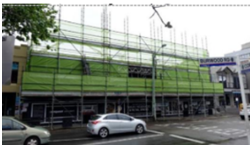
Example 15: Scaffolding Style – Not Acceptable in any zones
