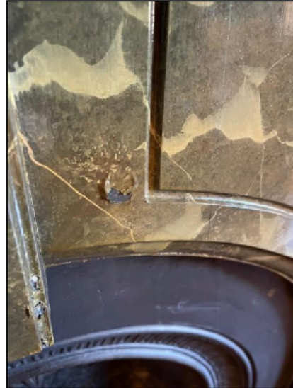
Figure 4. Detail of non-original fireplace on the ground floor, east wing of the residence. This view shows the bubbling plastic paint on the timber which has been made to look like marble. There are two of these fireplaces on the ground floor, in the living room and lounge room on the eastern side.
