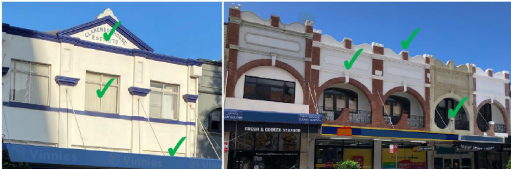
Figure 1(h). Examples of good quality facades without security bars, permanent grilles or air handling systems.
