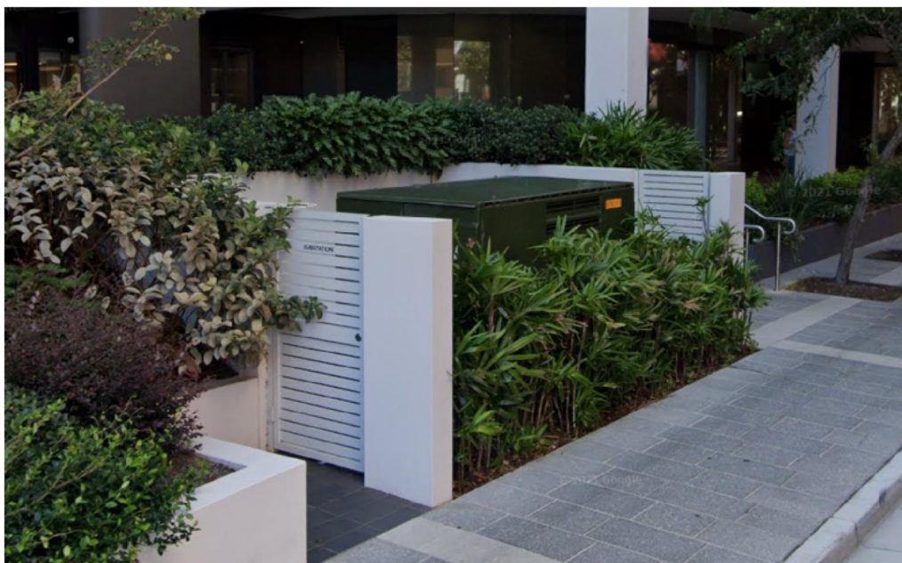
Figure 1(d): Example of a screened large power supply utility / substation
