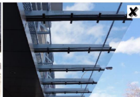
Glass awnings should demonstrate streetscape consistency and visual continuity with adjacent awnings.
