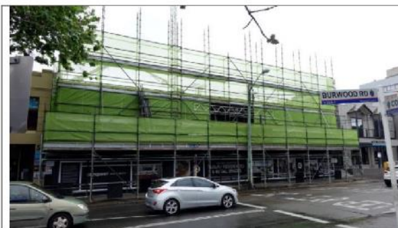
Example 15: Scaffolding style – Not Acceptable in any zone
