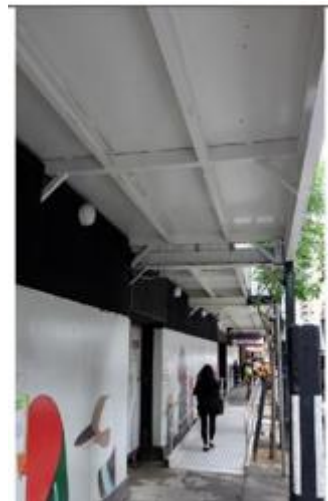
Example 14: Underside of hoarding must be painted white
