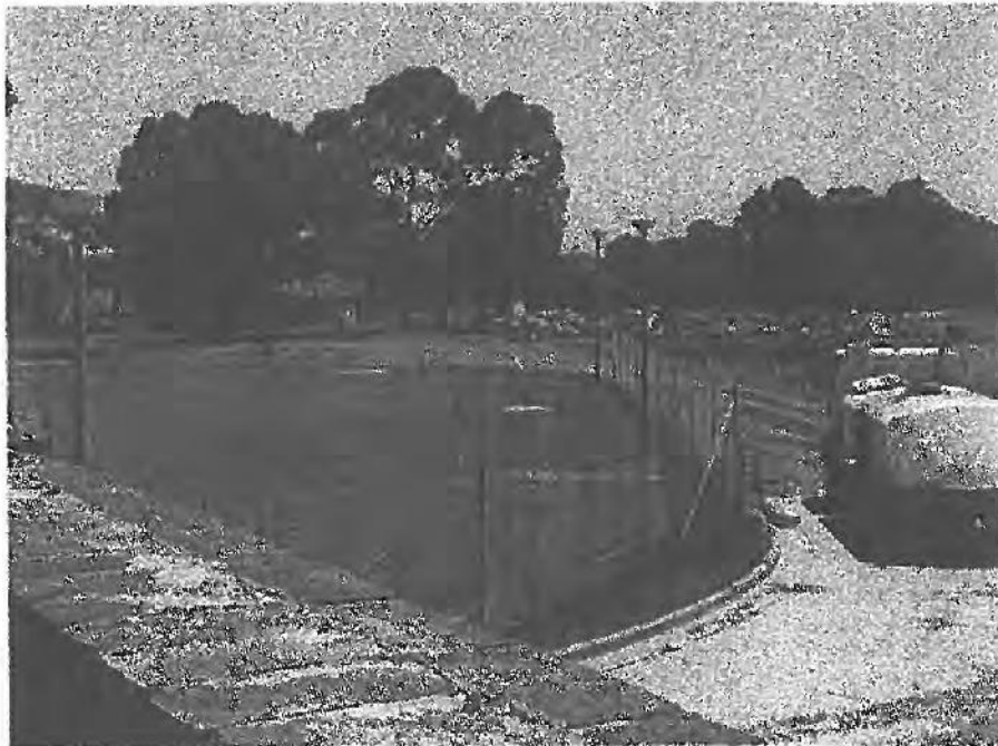
Photograph 2: Looking north west from retaining wall over the driveway showing remediated section.
