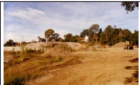
Figure S14 - Stockpiles of topsoil along the Blair Avenue boundary of the brickpit site, with completed ground works on the right. Photo: MWA 2005.
