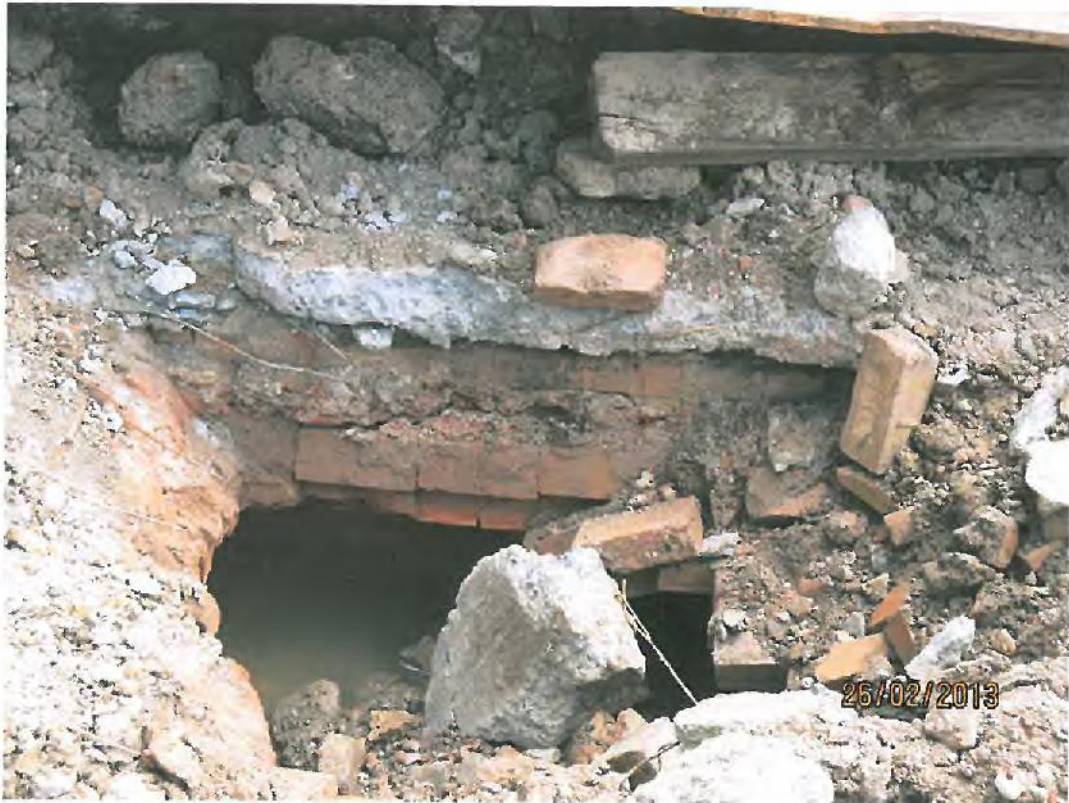
Figure 1: Section of flue with corbelled roof overlain by a concrete slab. Note brick to right with "B I" impression in frog.
