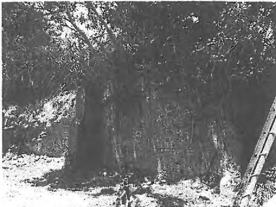
Photograph 4: Section of the brick retaining wall near adjacent to housing on the south east
